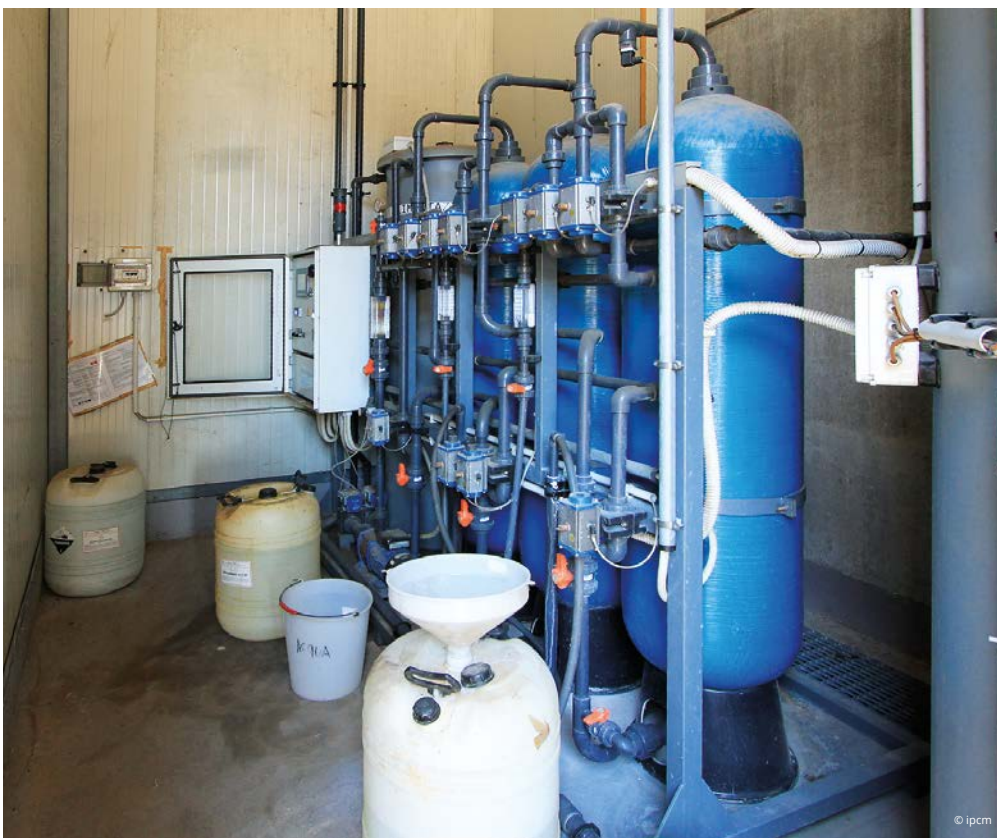
The pre-treatment tunnel with the tanks in the foreground and the demineralising columns.
