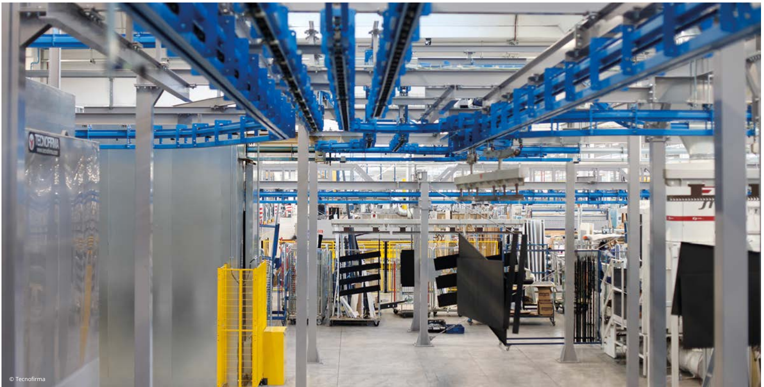
The Tecnofirma's coating system with the Futura's conveyor installed at ISA's plant.
