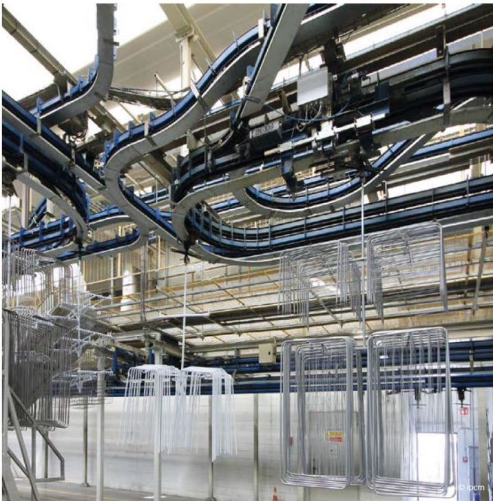
One of the most complex segments of the conveyor.
