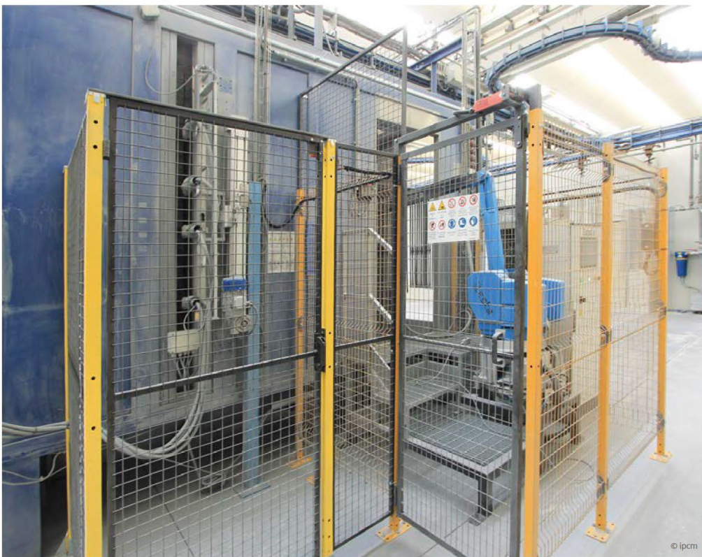
One of the coating booths with a Lesta articulated robot.
