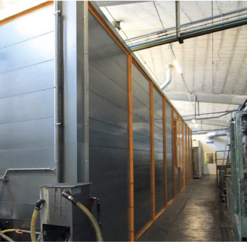
The new curing oven installed by Euroimpianti.
