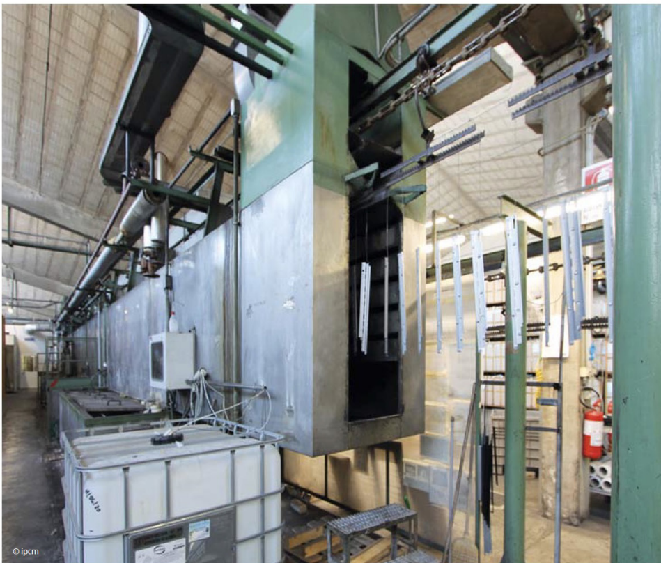
The pre-treatment tunnel.
