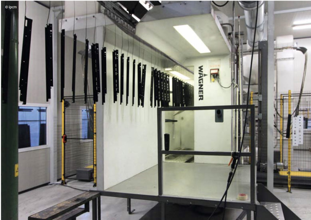
The new Wagner powder application booth.
